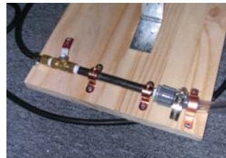
Figure 12.5. Reducing Fitting And Shutoff Valve
