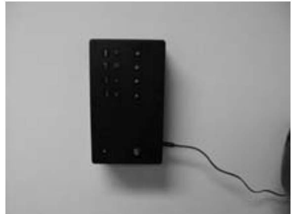
Figure 21.5. Nursing Station Unit Installed.
